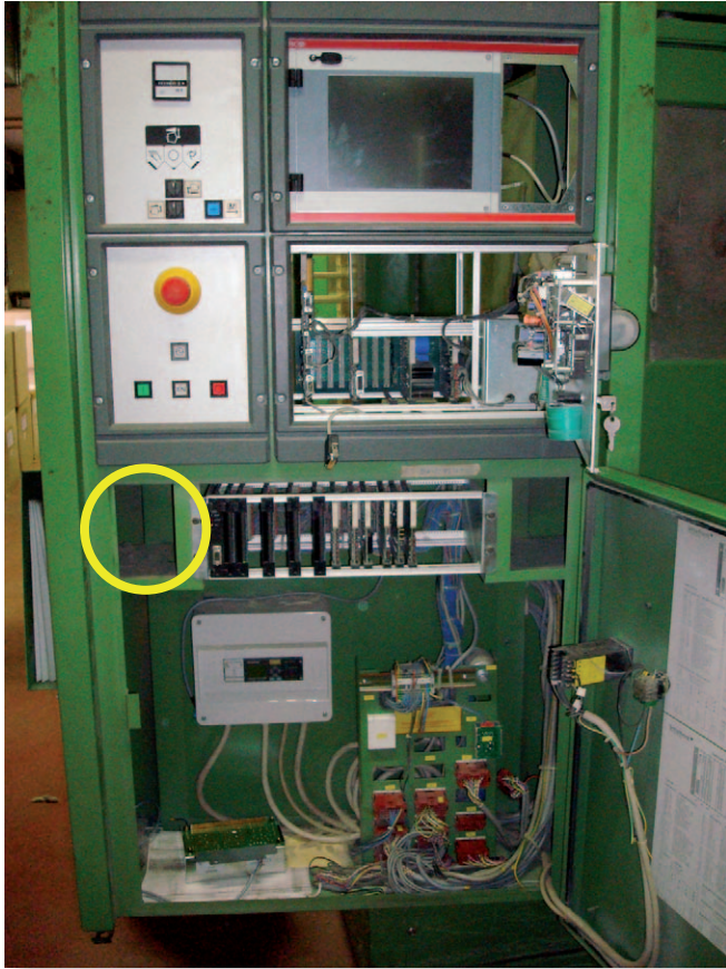
Cabling SCU Front
