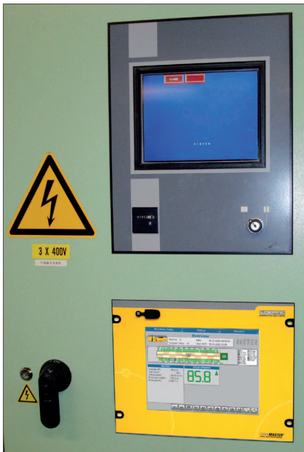
The SCU is installed in the headstock below of the Rieter PC.
