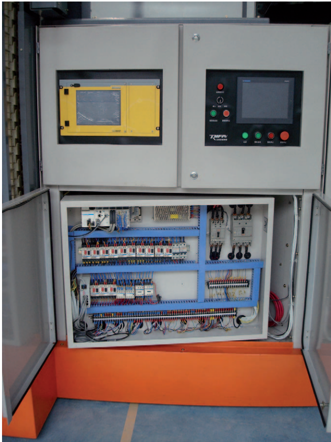
Cabling SCU Front
